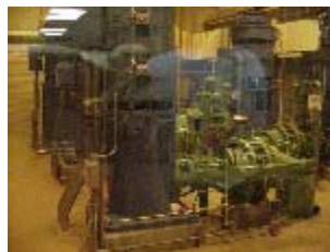
Pumps inside the Visitor Center.
