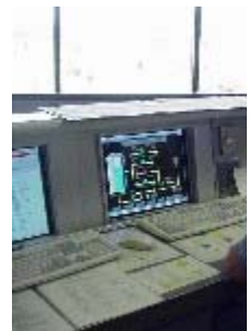
The control room is staffed 24 hours a day, 365 days a year.
